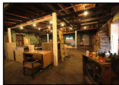
Before: Vacant commercial building and site of rental project in the City of Radford.
